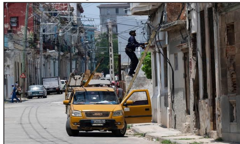
An electrician works on the power grid during a nationwide power outage in Havana.
