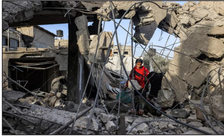
A woman and a girl search for items in the rubble of a collapsed building in Rafah in the southern Gaza Strip, on April 24, 2024, following Israeli airstrikes overnight.
