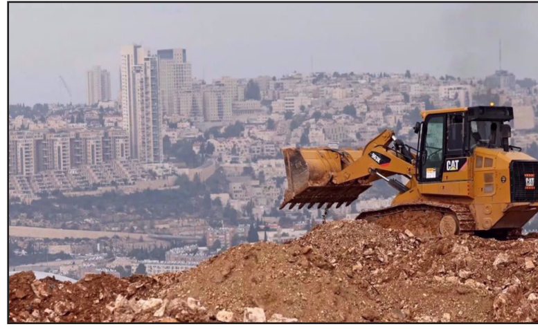
A bulldozer operates at a construction site near an Israeli settlement in East Al-Quds on December 7, 2023.
