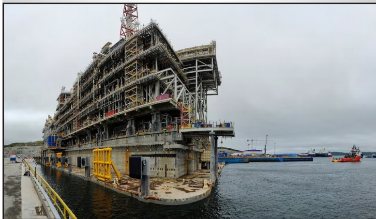
A view shows a gravity-based liquefied natural gas platform in the village of Belokamenka, Murmansk Region, Russia July 20, 2023.
