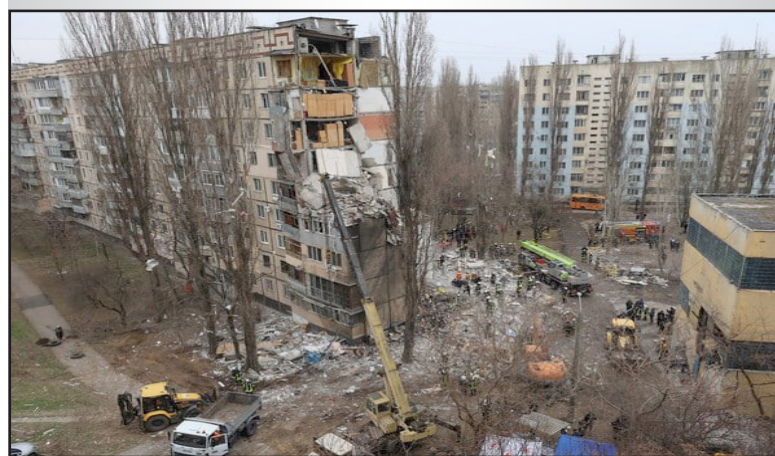
Rescue crews working at the site of a residential building heavily damaged by a drone strike that killed several residents, in Odesa March 2, 2024.
