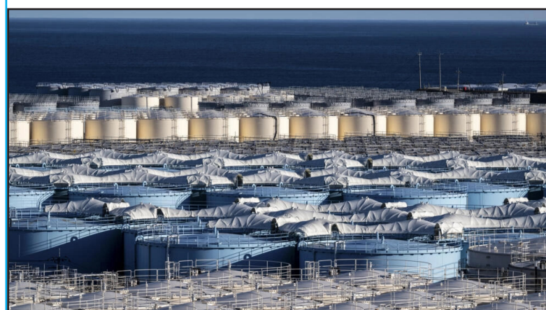
Storage tanks for contaminated water at the Tokyo Electric Power Company's (TEPCO) Fukushima Daiichi nuclear power plant, Okuma, Fukushima prefecture, January 20, 2023.
