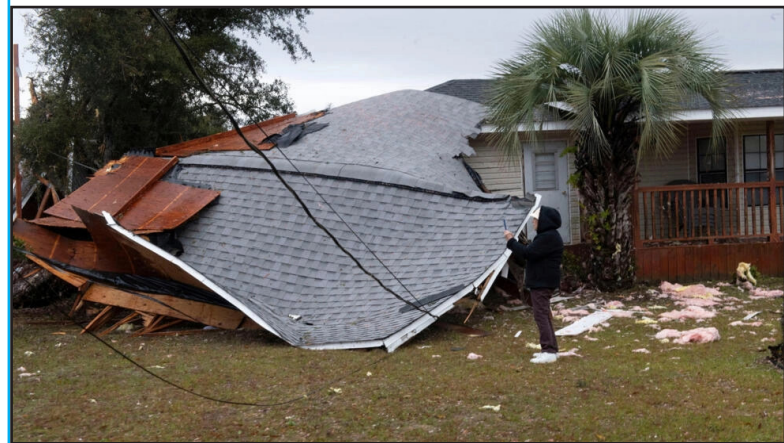
A resident checks a collapsed roof after a line of storms roared through the area of Perdido Key near Pensacola, Florida, U.S. January 9, 2024.
