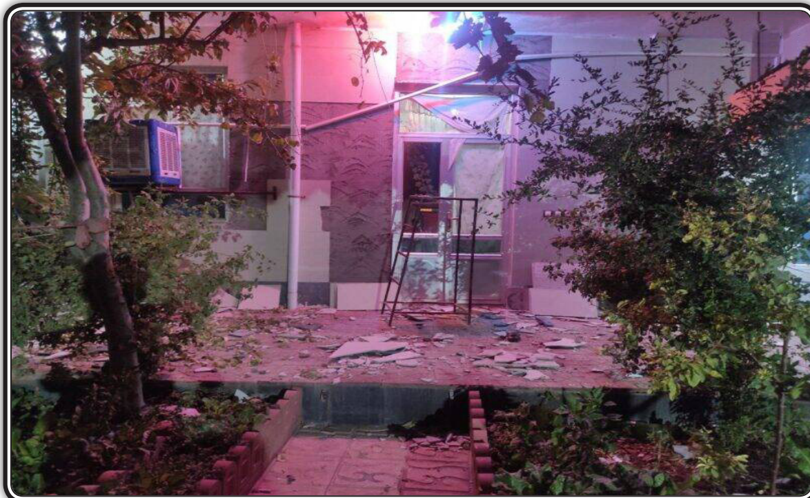
The quake on Wednesday caused cracks in buildings in Khoy and other cities.
