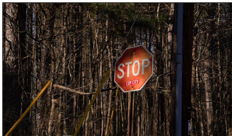
A stop sign sits on the outside of the forest as construction continues after a SWAT escort this morning at the construction site of a public safety training facility that activists have derided with the nickname "Cop City", in Atlanta, Georgia, U.S., February 6, 2023.
