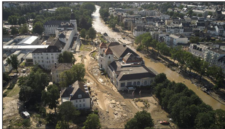
Damage and debris from flooding is near the Ahr River, including in the spa complex, Sunday, July 18, 2021, in Bad Neuenahr, Germany.
