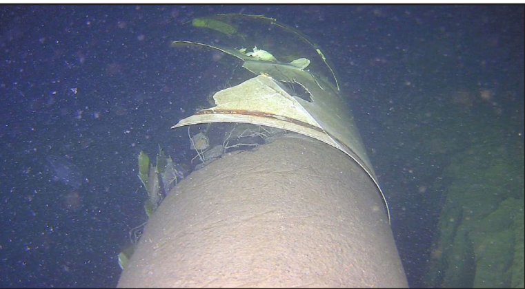
Damage is seen to the Balticconnector gas pipeline that connects Finland and Estonia across the Baltic Sea.
