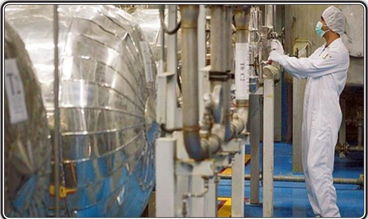
(File photo): A technician checks valves at the uranium conversion facility
