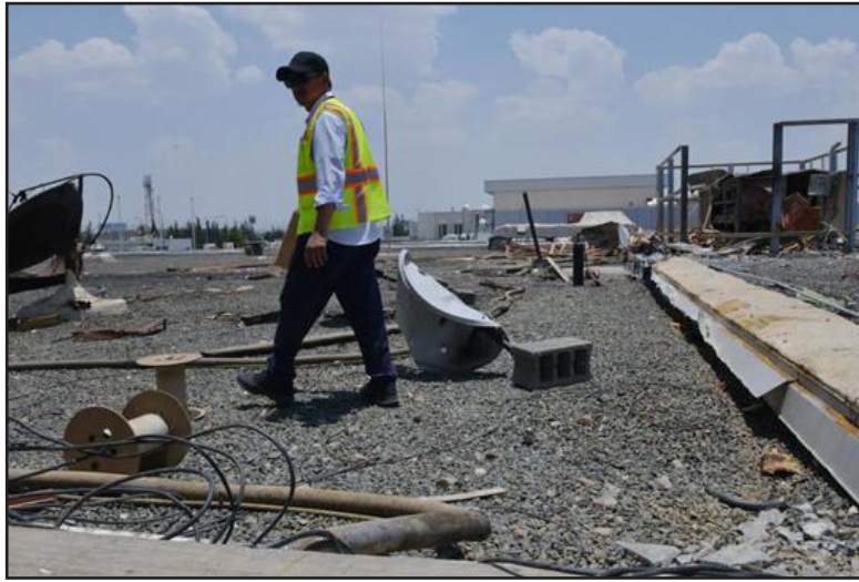
A worker is inspecting the damage at Abha airport in Saudi Arabia, one day after a missile attack by Yemeni armed forces and their allied fighters from Popular Committees.
