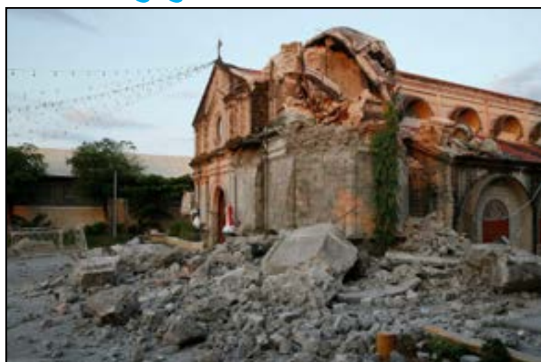
Damaged St. Catherine church is seen following a 6.1 magnitude earthquake that also caused the collapse of a commercial building in Porac township, Pampanga province, north of Manila, Philippines, Tuesday, April 23, 2019.
