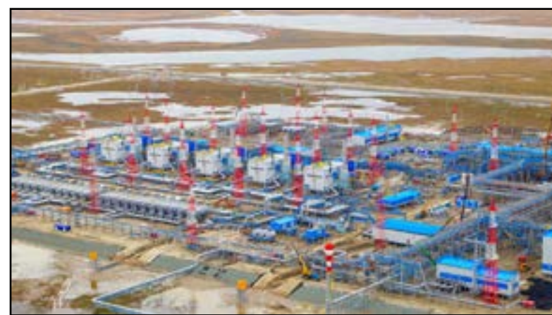
Gas production facility No. 3, Bovanenkovo gas field
