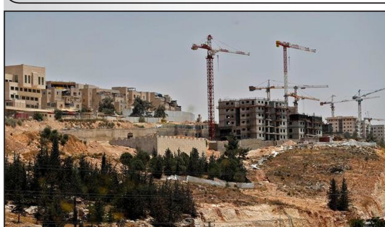
A picture taken on July 24, 2018 shows a view of ongoing construction work at Ramat Shlomo, a settlement in the mainly Palestinian eastern sector of al-Quds.
