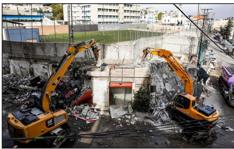
This picture taken on November 21, 2018 shows two excavators of the al-Quds municipality, demolishing one of over a dozen shops in the Arab-inhabited Shuafat refugee camp in Israeli-annexed East al-Quds, which Zionist regime authorities said were built without a permit.
