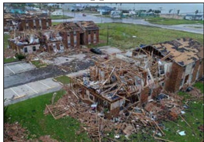
Aerial footage shows damage to Salt Grass Landing Apartments in Rockport, Texas, after Hurricane Harvey.
