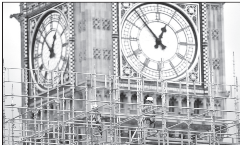
Construction work is carried out on the Elizabeth Tower, commonly known as Big Ben, in London on July 4, 2017.
