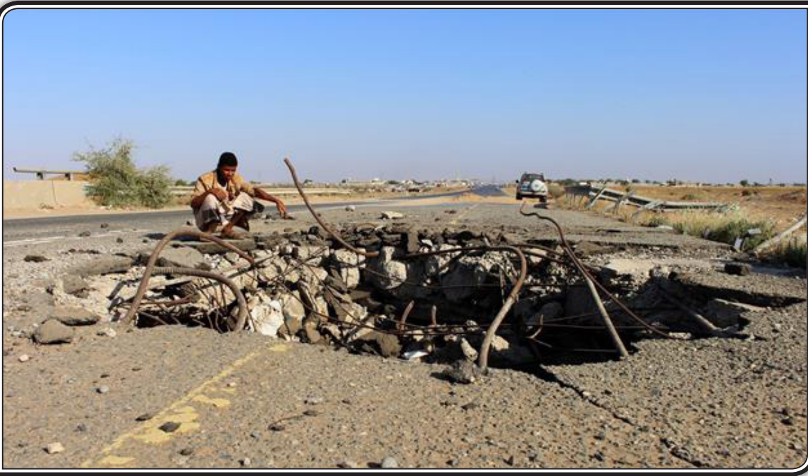
A Yemeni man inspects the damage made by a Saudi airstrike on a bridge between the area of Abbas and Harad in the northern province of Hajjah, on December 25, 2017.
