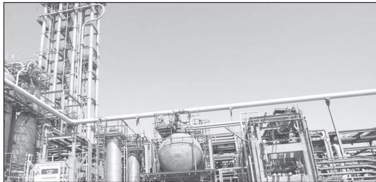
A view of the Mahshahr petrochemical plant in the southwestern Iranian province of Khuzestan.
