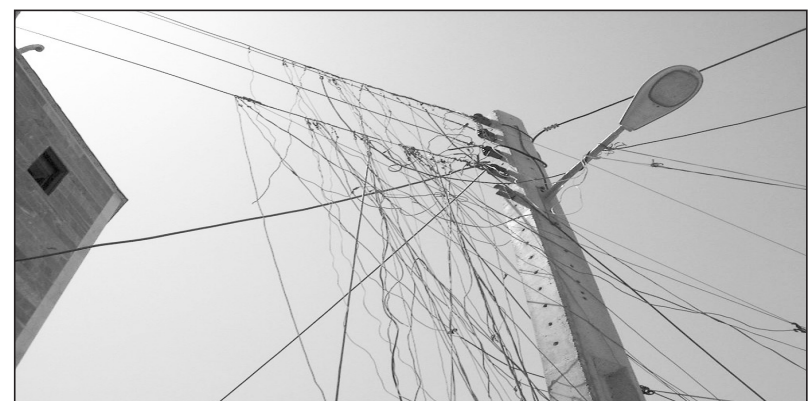
The illegal use of power from local utility lines
